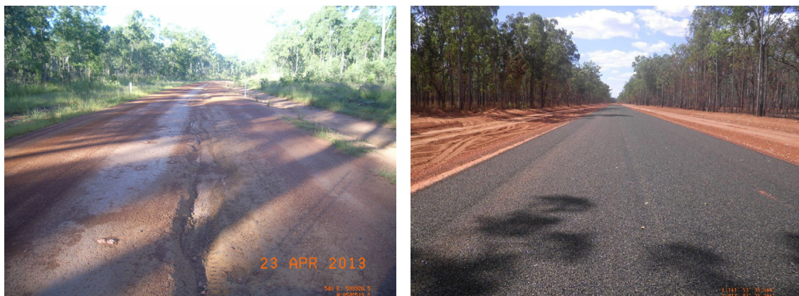
Figure 4: Aurukun Access Road (the only road link to and from the Aurukun community). Left: Gravel road that was damaged in 2010, 2011, 2012 and 2013. Right: Bitumen seal instated in 2013 along a 10 km vulnerable section. This has since withstood the impacts of eight natural hazard events (photos courtesy of QRA).
