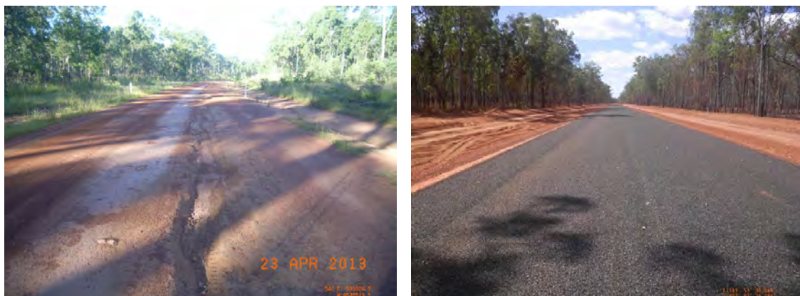
Figure 4: Aurukun Access Road (the only road link to and from the Aurukun community). Left: Gravel road that was damaged in 2010, 2011, 2012 and 2013. Right: Bitumen seal instated in 2013 along a 10 km vulnerable section. This has since withstood the impacts of eight natural hazard events (photos courtesy of QRA).
